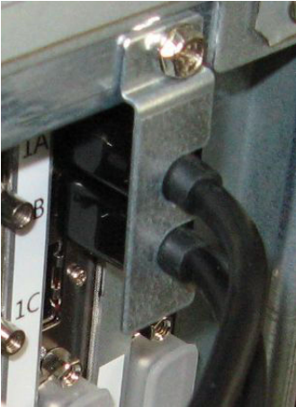
Fig. 2: Installed holder with DP connectors
